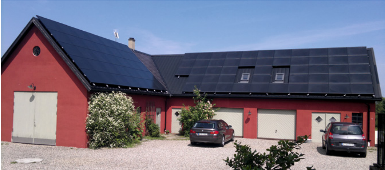
On the roof of a former farm in Simrishamn, southern Sweden, 84 Solar Frontier CIS thin-film modules were installed facing south-east and south-west. (Image: Futura Energi)
